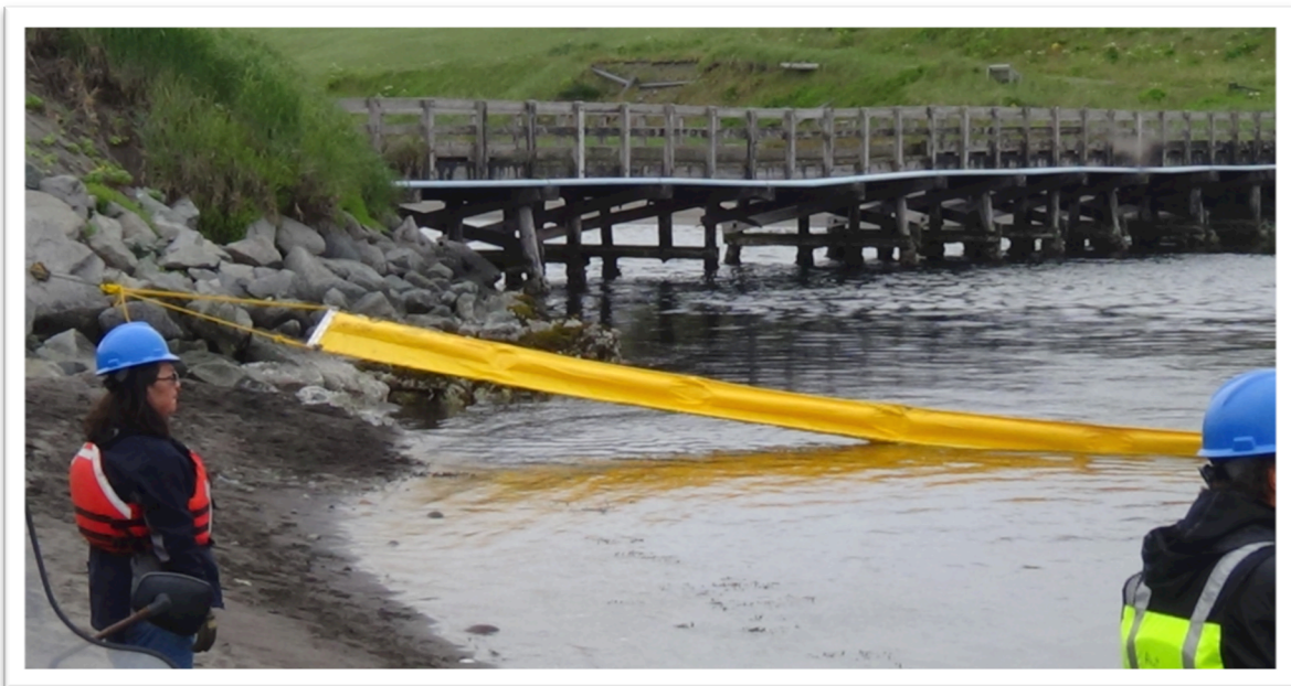
Figure 7. Crews had difficulty with shore anchor systems
